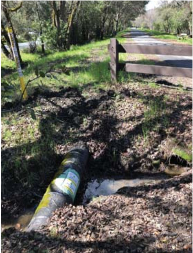
Exposed high transmission gas pipeline along the Lafayette Moraga trail.
